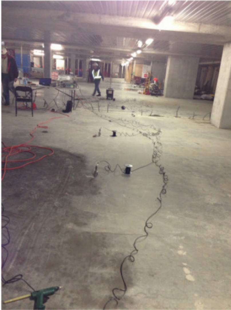
View of test setup from Eastern to Western test spans (EMA testing)
