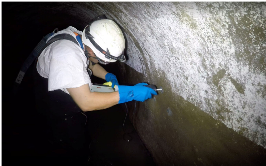
Figure 3. Measurements of the pH levels in concrete pipe linings on-site for evaluations of the state of acid permeation [10].
